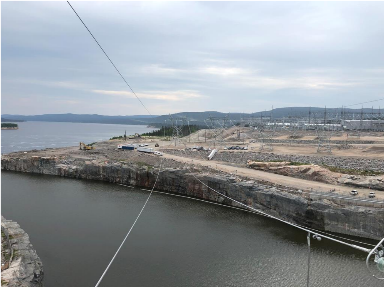
Photo 4 - Four interconnecting lines between the Powerhouse and Converter building
