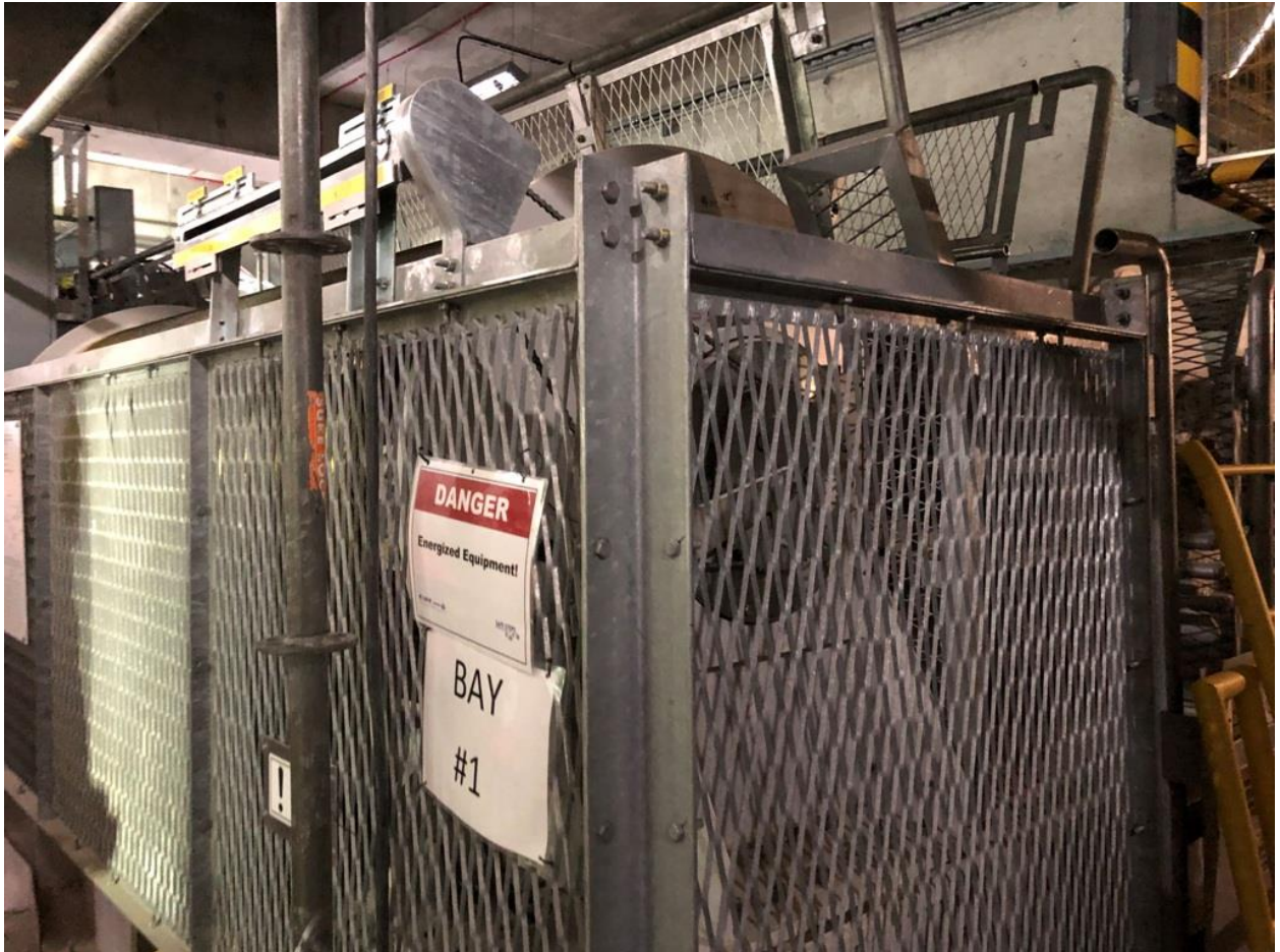
Photo 5 - Intake gate hoist
