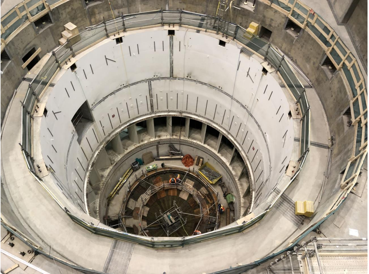
Photo 9 - Unit 4 Turbine pit and stay ring
