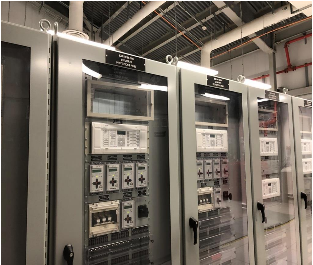
Photo 1 - SOP Convertor building switchboards
