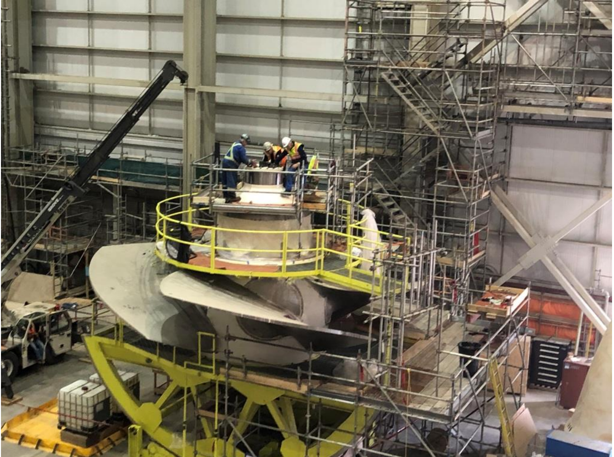
Photo 8 - Unit 2 Turbine runner
