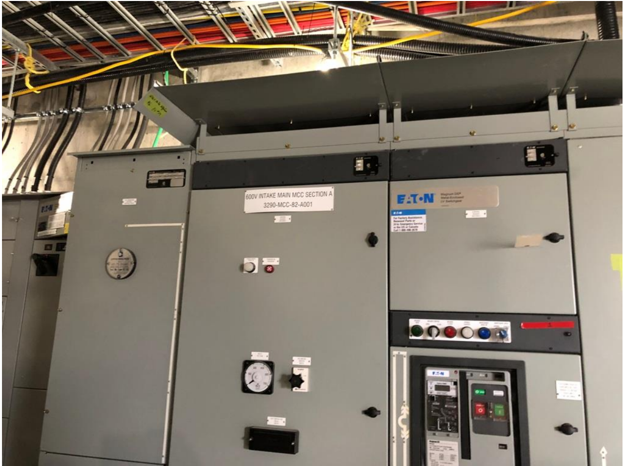
Photo 6 - Intake gate hoist Motor Control Centre (MCC) detail
