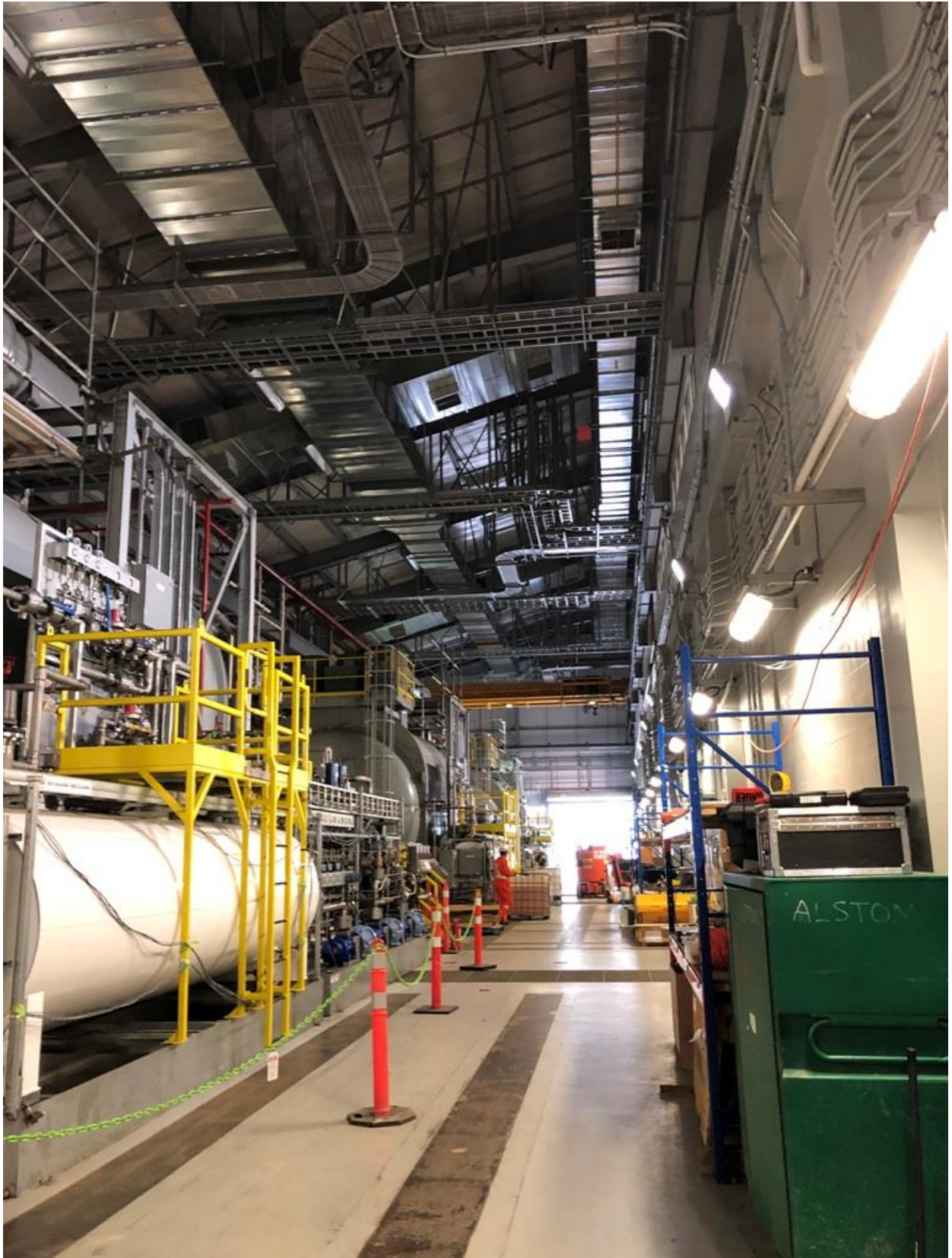
Photo 2 - SOP Synchronous Condensers building
